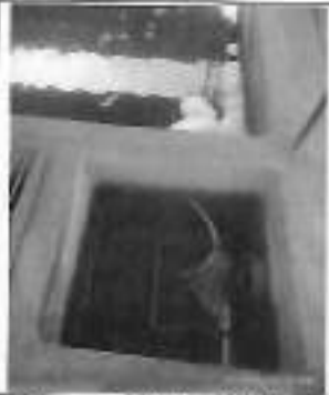
Photo 19: Inlet Collection tank
