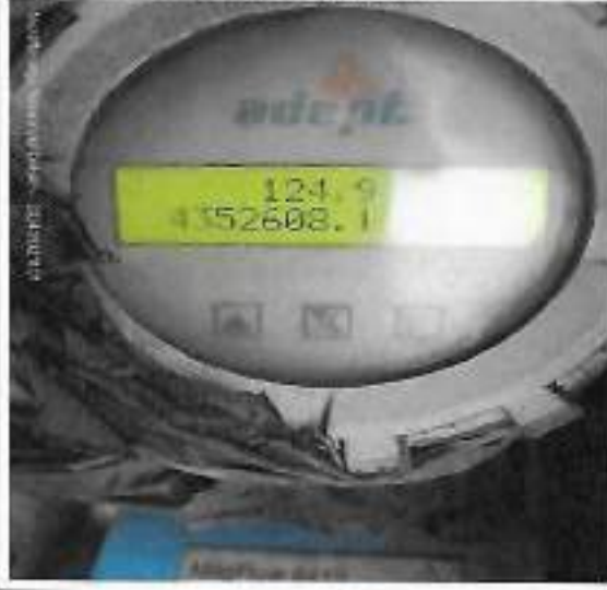
Fig.7: Flow meter at recycling line
