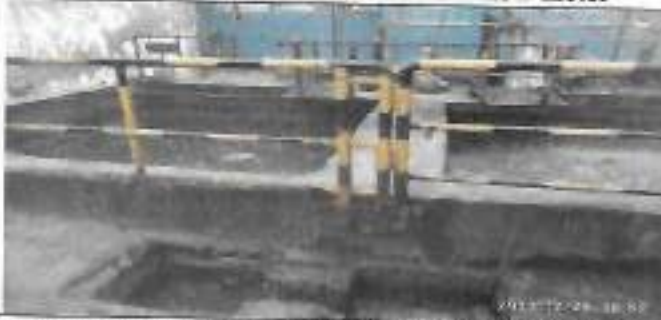
Photo 4: ETP inlet collection tank (High COD & Low COD)
