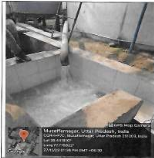
Flow meter installed at Borewell No. 2
