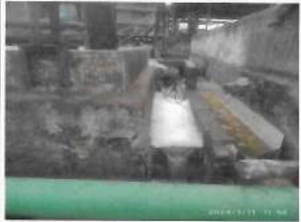
ETP outlet channel
