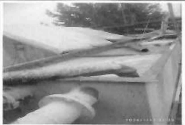
Storage tank for recycle after equalization
