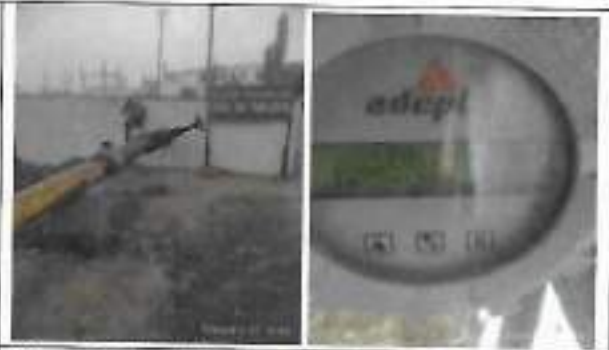
Photo 2: ETP inlet line with flow meter
