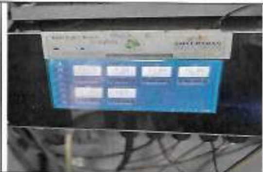
Photo 10: OCEMS at ETP outlet
