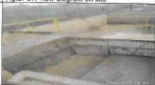
Fig.4: Inlet screen and equalization tank
