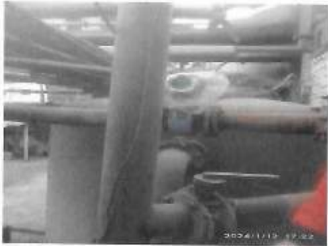
Flowmeter at ETP recycling line (after ACF)
