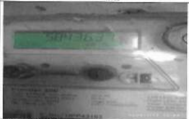
Photo 13: ETP energy meter
