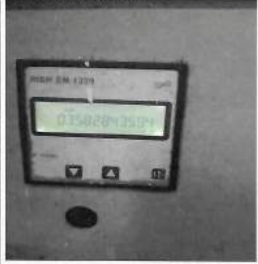
Fig.8: ETP energy meter
