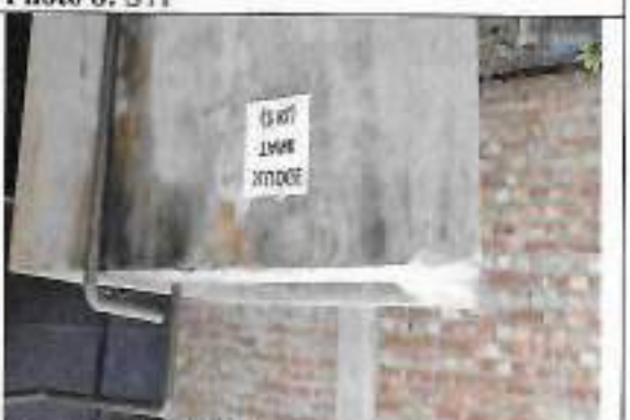
Photo 10: STP Sludge tank
