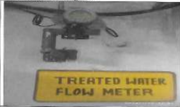
Photo 11: ETP outlet flow meter
