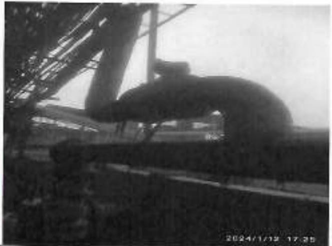
Flowmeter at ETP recycling line (after primary clarifier)
