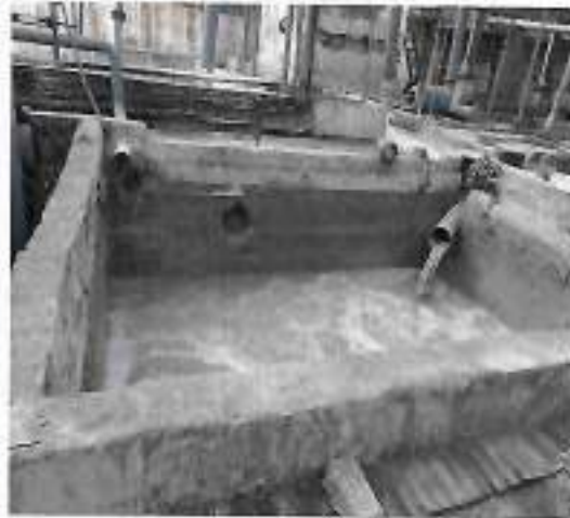
ETP collection tank
