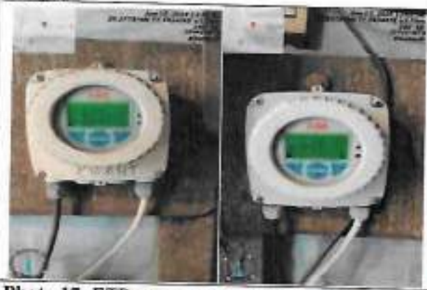
Photo 17: ETP energy meter with reading
