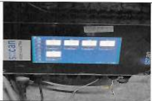
Fig.12: OCEMS at ETP outlet
