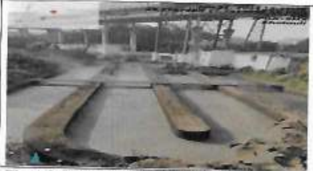
Photo 8: ETP Units (Secondary clarifier)
