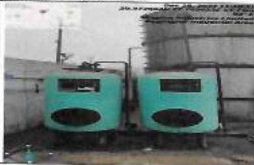
Photo 9: Filtration units for tertiary treatment
