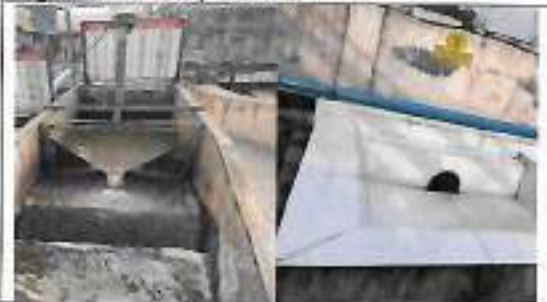
Fig.7: ETP Outlet, v-notch and ultrasonic meter
