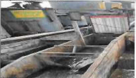
Fig.7: ETP Outlet, v-notch and ultrasonic meter
