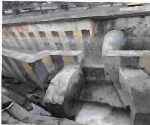
Outlet of secondary clarifier
