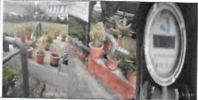
Photo 2: Borewell -1 & 2 with common flow meter
