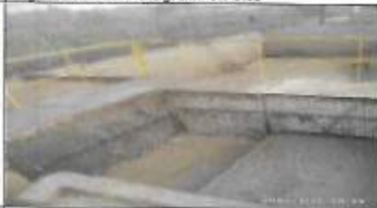
Fig.4: Inlet screen and equalization tank
