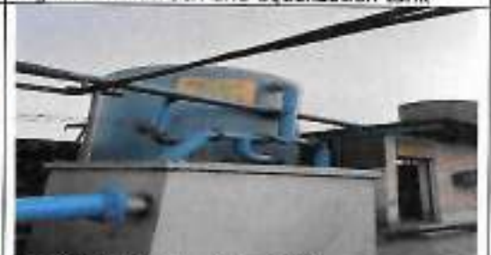
Fig.6: Multi Grade Filter (MGF)
