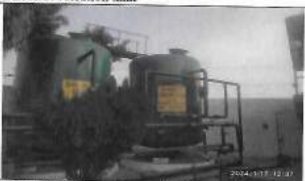
Photo 7: Tertiary treatment (DMF + ACF)
