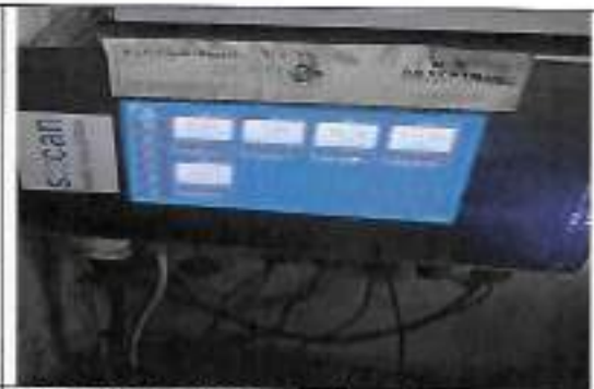
Photo 10: OCEMS at ETP outlet
