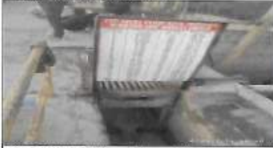
Fig.3: ETP inlet (v-notch and ultrasonic meter)
