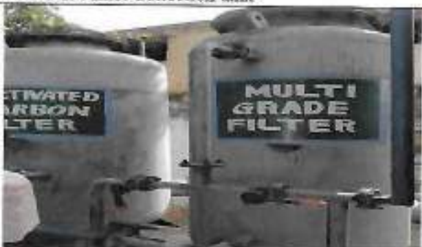
Photo 21: Filters in STP
