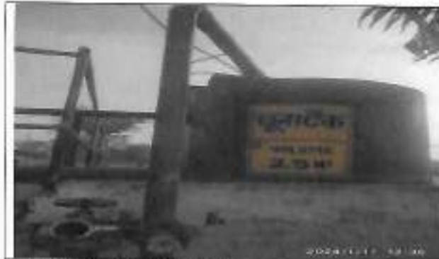
Photo 9: Lime dosing tank
