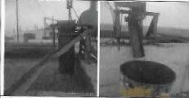
Photo 3: Oil &amp; Grease tank with skimmer
