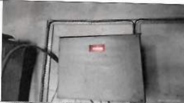
Photo 7: ETP inlet Flowmeter with reading
