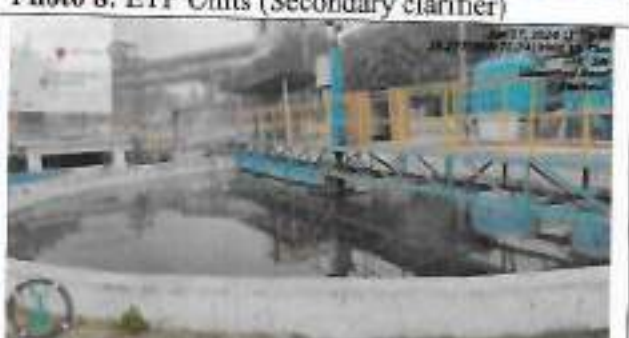
Photo 10: STP Units (Clarifier)
